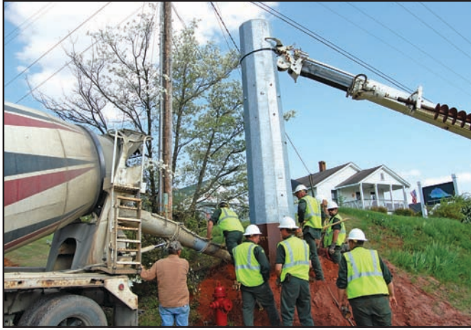
Blue Ridge Mountain EMC crews install a new transmission line. Photo by Lowell Nicholson
