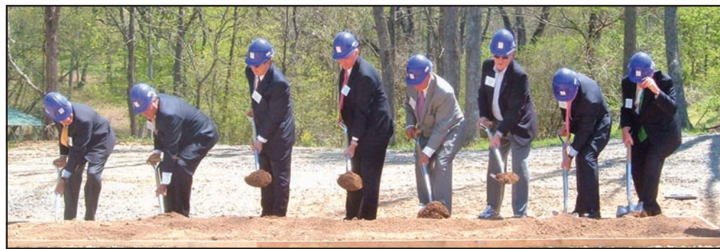
Members of the Board of Trustees broke ground on Friday for a new 57,000 square foot recreation center that will open in the summer of 2010. Photo by David Seckinger
