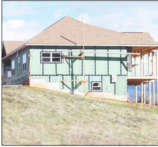
A new home going up is a rare site in Towns County these days. Actually, this could soon be a sign of the times. Photo/Joe Collins
