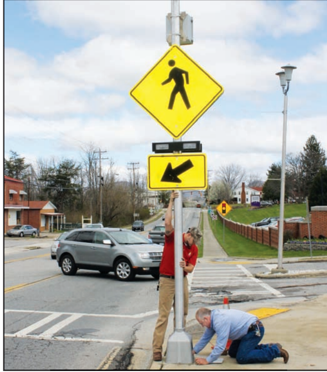
Mark Zinn and Eric Richards install the new crosswalk beacons across from Young Harris College. It's an attempt to save lives. Photo/Libby Shook
