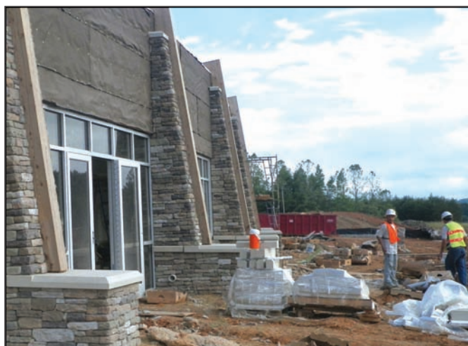
Workers finish outside work at the new Towns County Recreation Center on Mining Gap Road. Photo/Joe Collins
