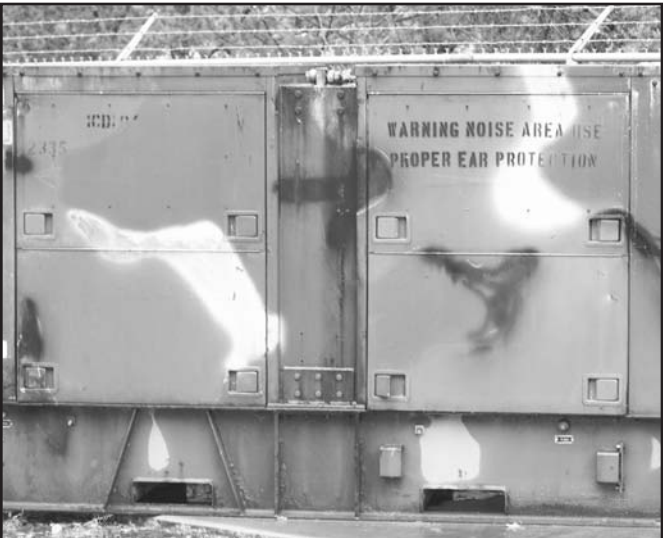
The newest generator replaces this Vietnam-era model that is now retired from service. Photo/Shawn Jarrard
