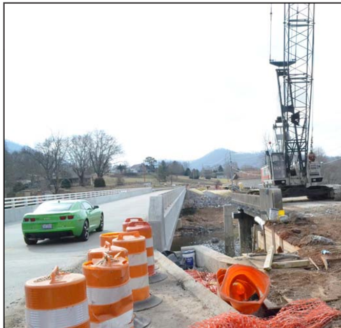
The new High Bridge is open, and the old bridge is almost history. Photo/Lowell Nicholson
